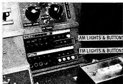
Fig. 1. Control panel placed in console.
